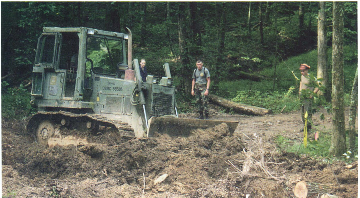
Company D, 4th CEB build a road as a community service project during annual training in Rookwood, TN.
