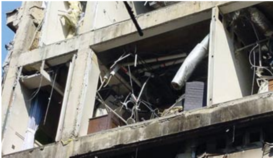
Outside view of damaged Marine Corps office spaces.
