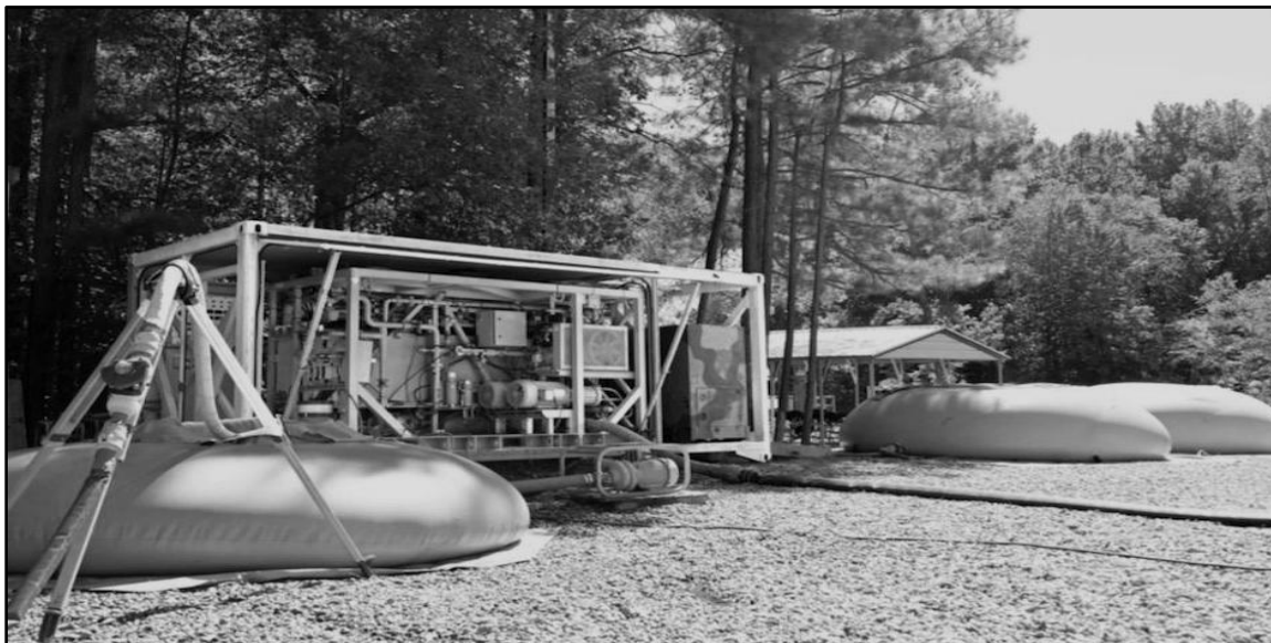
Figure A-2. Tactical water purification system
