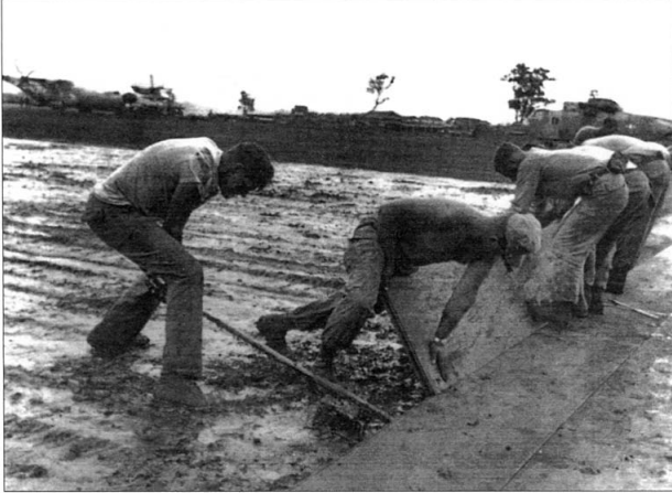
Seabees of Mobile Construction Battalion-301 set and seal aluminum runway mats into place at Khe Sanh Combat Base.
